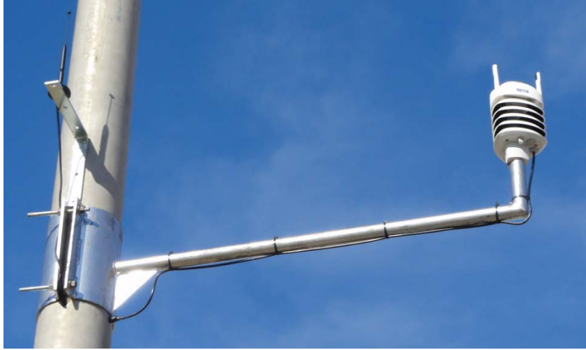
Figure 6: RWIS located in Siloam Springs
