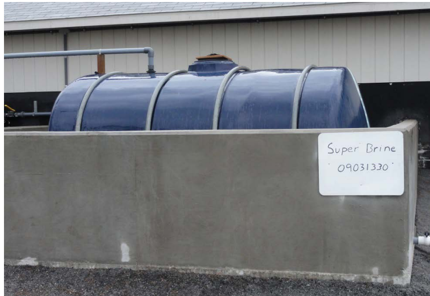
Figure 3: District 9 Super Brine Mixture Tank
